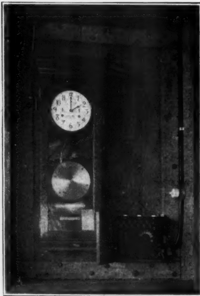
Clock Which Controls the Automatic Stokers.
